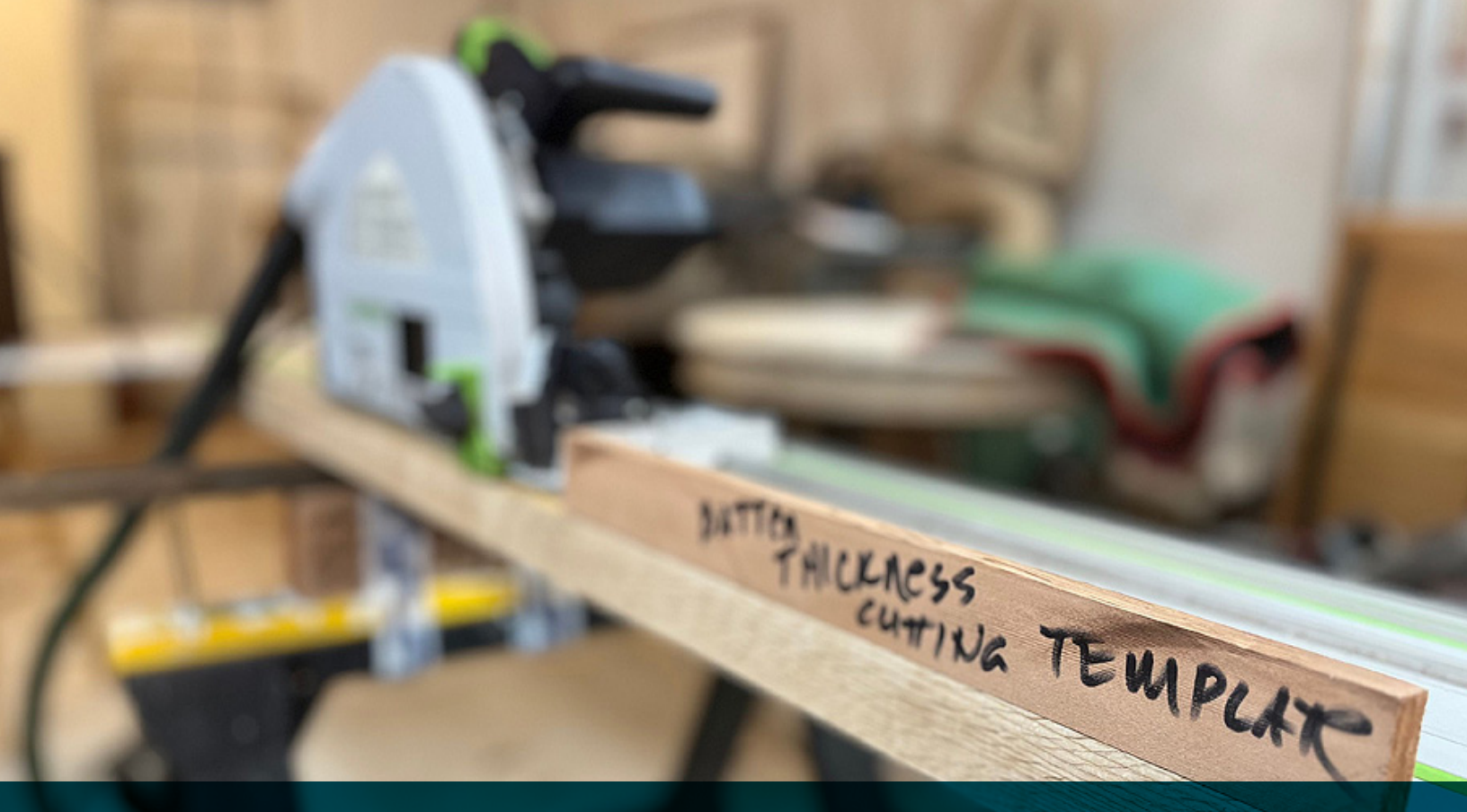
A track saw was used to cut the keel and battens, helping to ensure straight cuts and proper width
